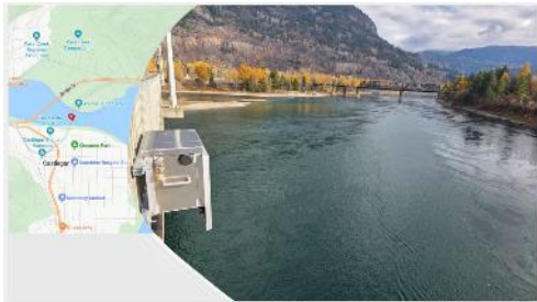
Columbia River below Norns: Water Level Gauge
